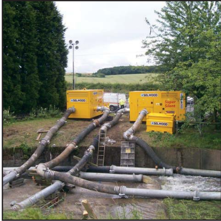
Flood Control (UK)
