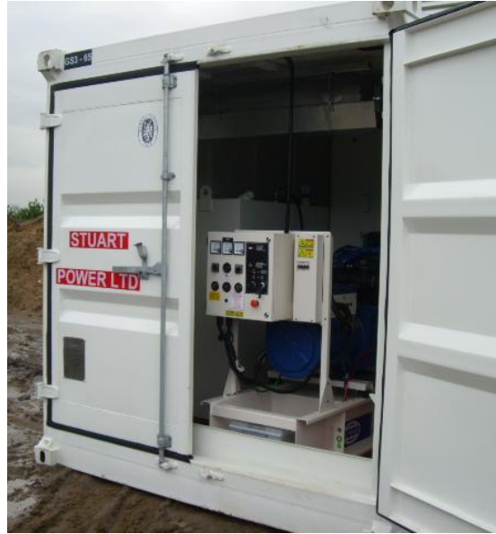
Twinpak showing upfit with single 65kVA generator (Rental Fleet Application)
