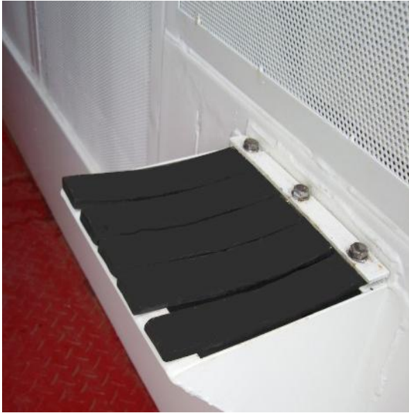
Cable entry point – anti vermin
