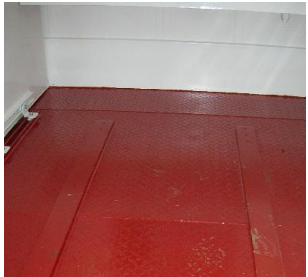
Bunded floor to contain fluids
